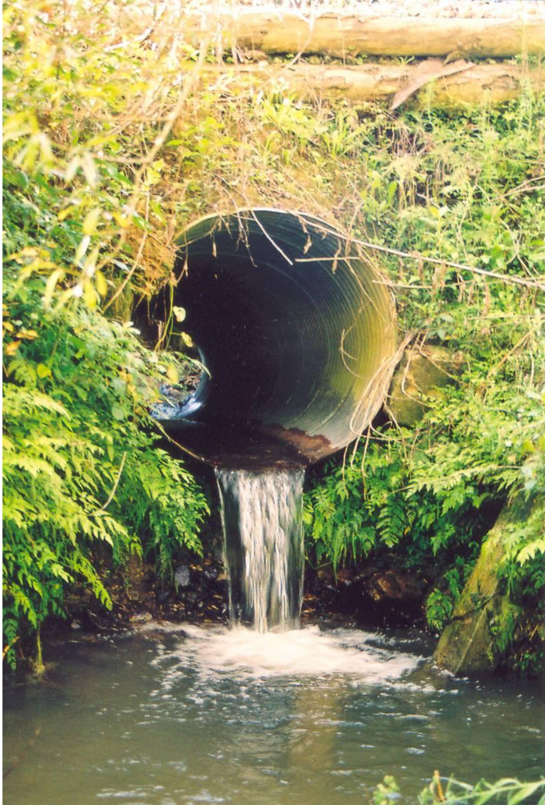
This culvert under a driveway across a small Pohara stream completely eliminates the passage of most native fish because it overhangs both the water and surrounding wet ground. It needs a rock or concrete ramp up which poor climbers like inanga can swim.
